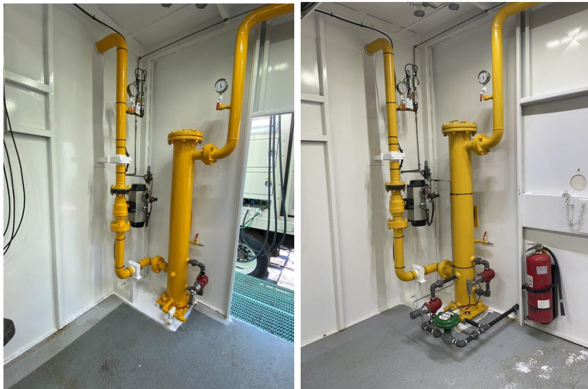
Figure 22: Before and After Automatic Dump Valve Installed on Engine Fuel Gas Scrubber
