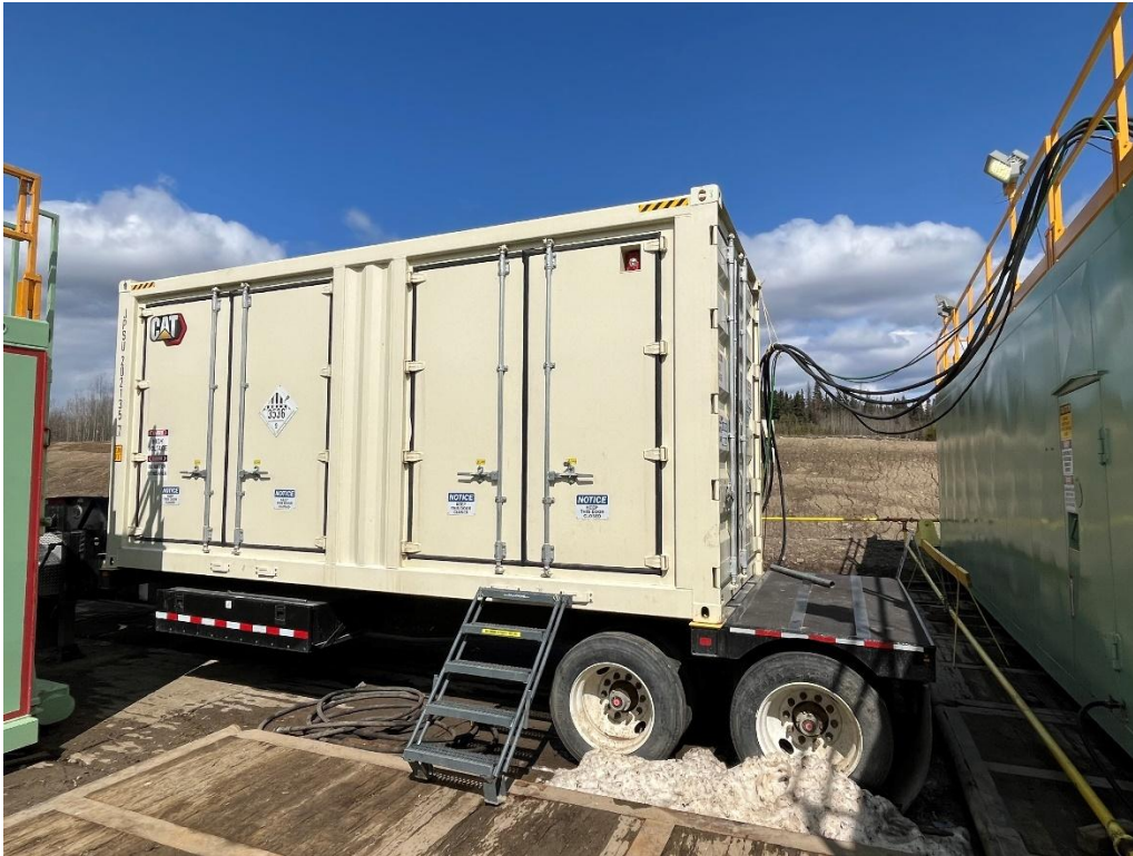
Figure 3: ESS Container and Trailer
