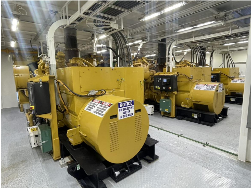
Figure 2: Inside of the Natural Gas Generator Building
