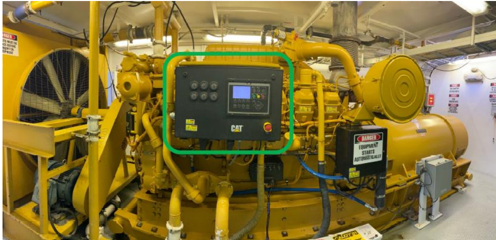
Figure 9: Project Rig #1 Upgraded EMCP 4.4 DGB Unit
