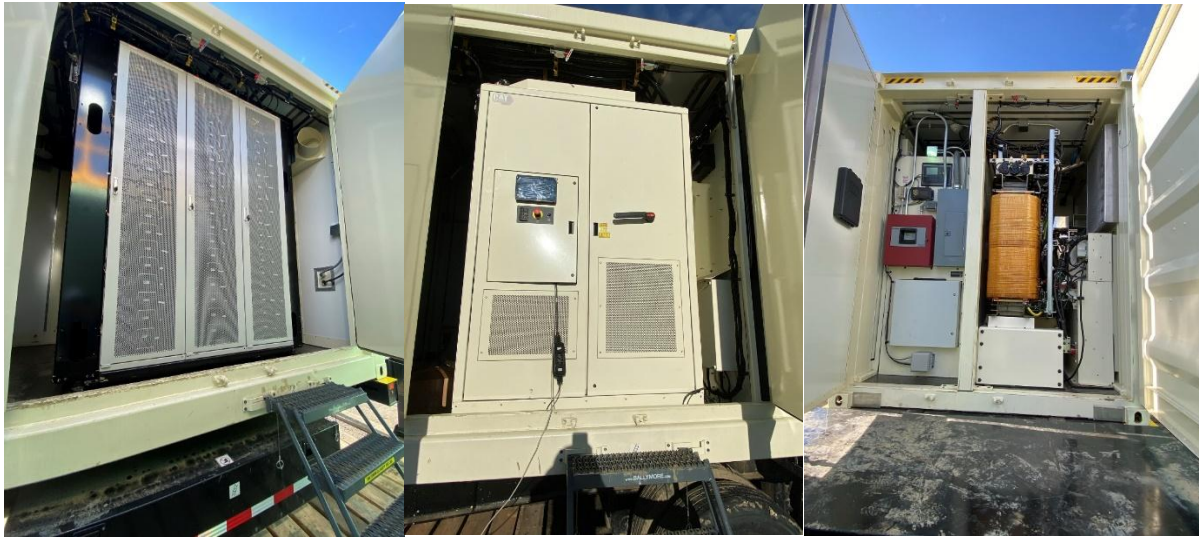
Figure 13: Inside View of ESS at Project Rig #1
