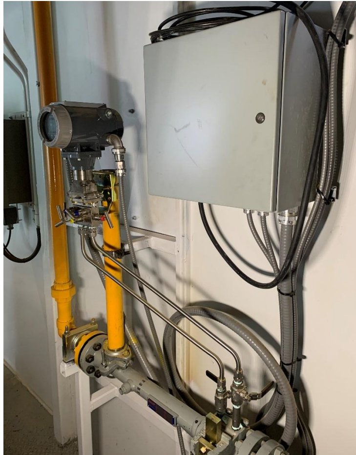
Figure 14: Natural Gas Flow Measurement on Project Rig #1
