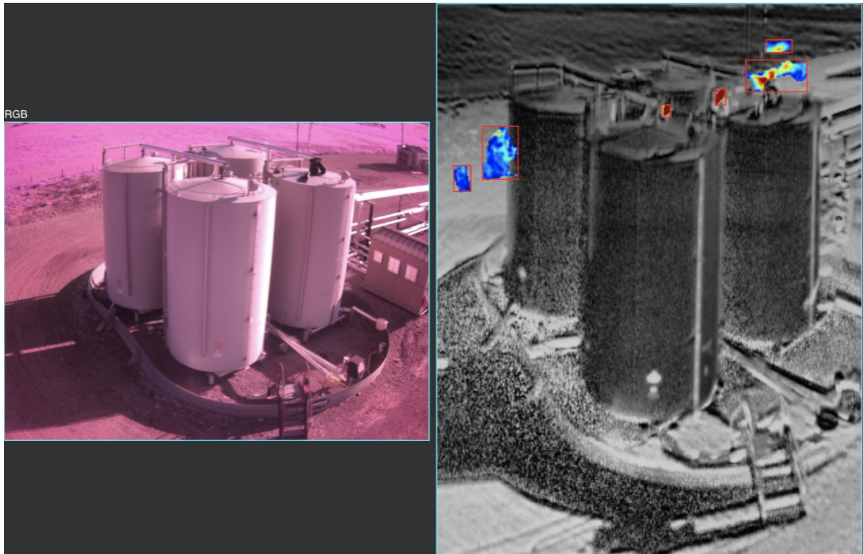
Figure 3-22 Emissions from Controlled Tanks Before Repair
