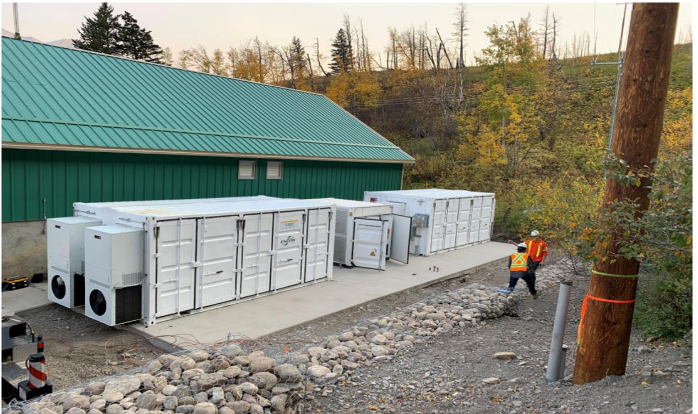
Figure 3: Waterton Microgrid BESS System
