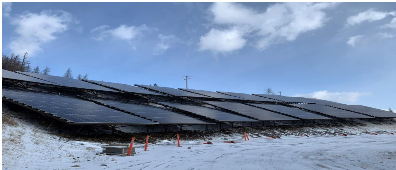
Figure 2: Waterton Microgrid Solar PV System
